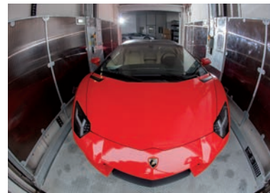
Internal view of one of the car lifts with polycarbonate side guards.
